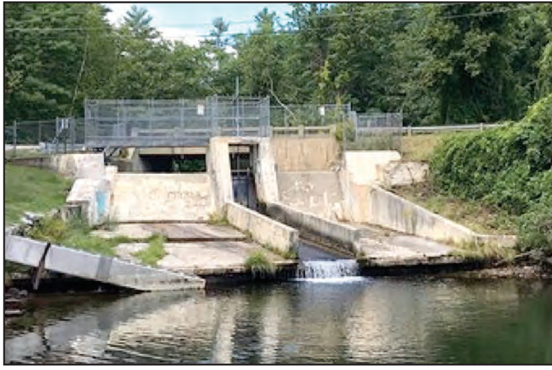
The Mill Street Dam in Raymond will be undergoing restoration starting June 1 and running through September 1. All work will be performed on the downwater side of the bridge heading from Main Street to Route 85. SUBMITTED PHOTO
